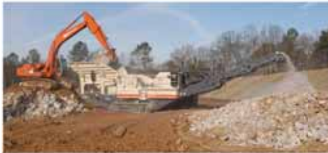
Portable Rock Crushing Plant
